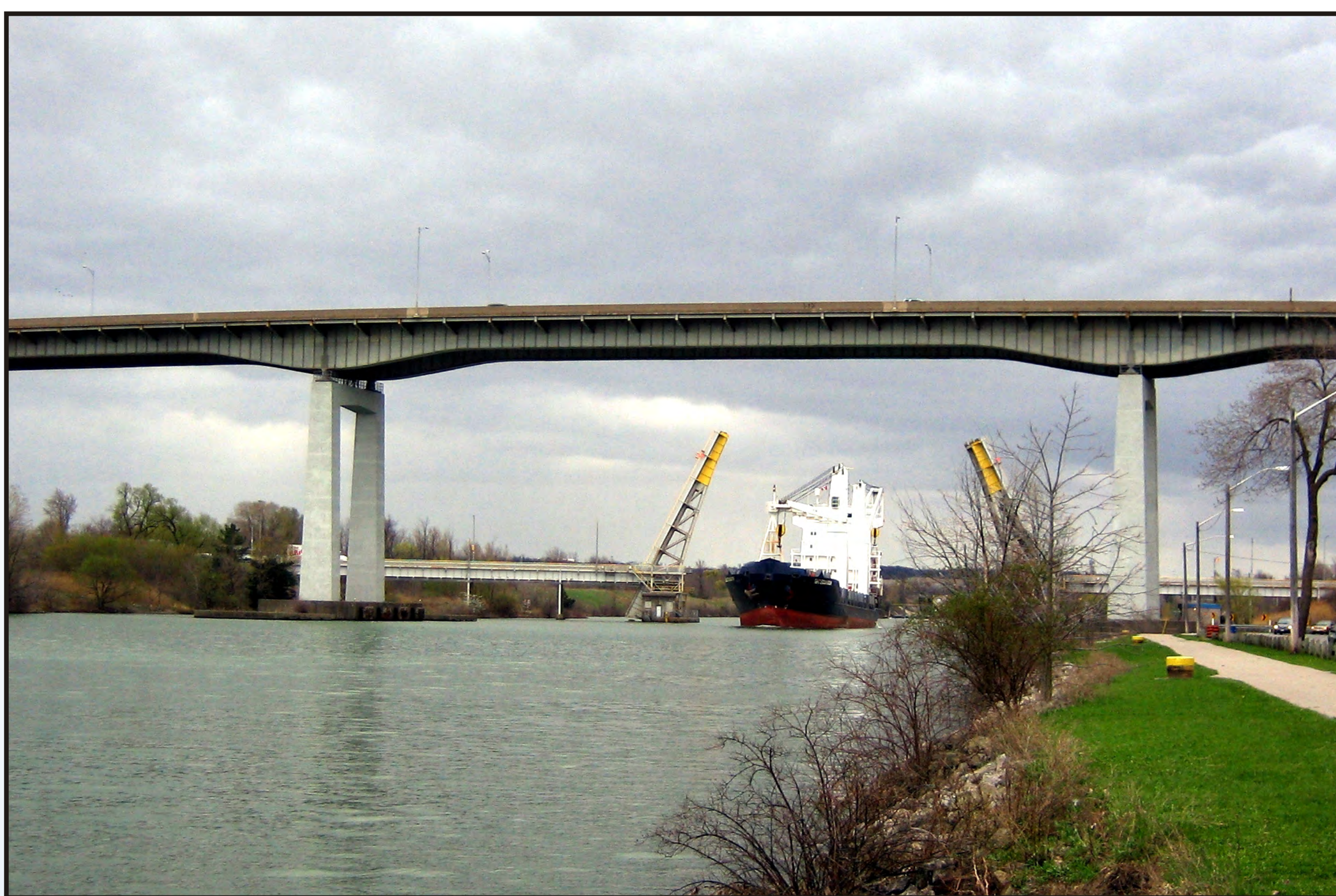
Looking south at the Garden City Skyway. In the background, a ship transits the Homer Bridge
